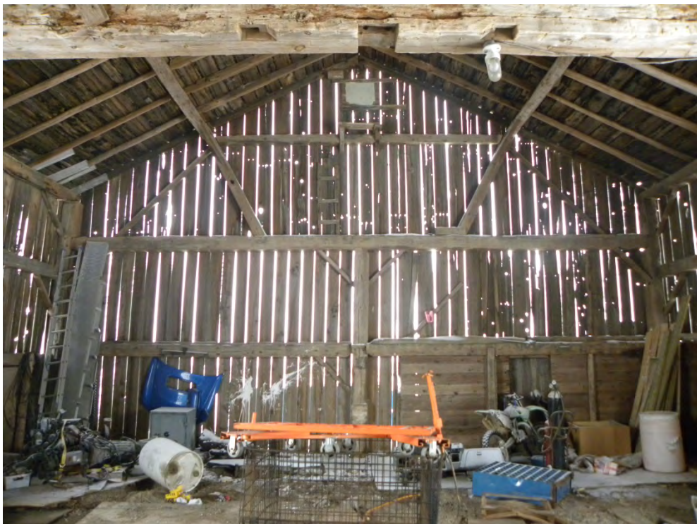
Plate 21: Interior west wall showing a typical timber-frame bent used as an end wall for barn construction. Two horizontal cross beams are located on this bent supported by a central vertical post. The lower cross beam consists of two short spans
