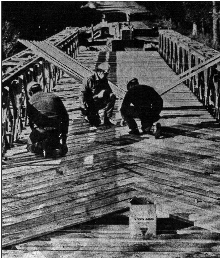
Figure 5. A view across the bridge shows the completed Bailey bridge structure and the wood plank deck laid in a herringbone pattern [ Guelph Mercury , October 16, 1974].
