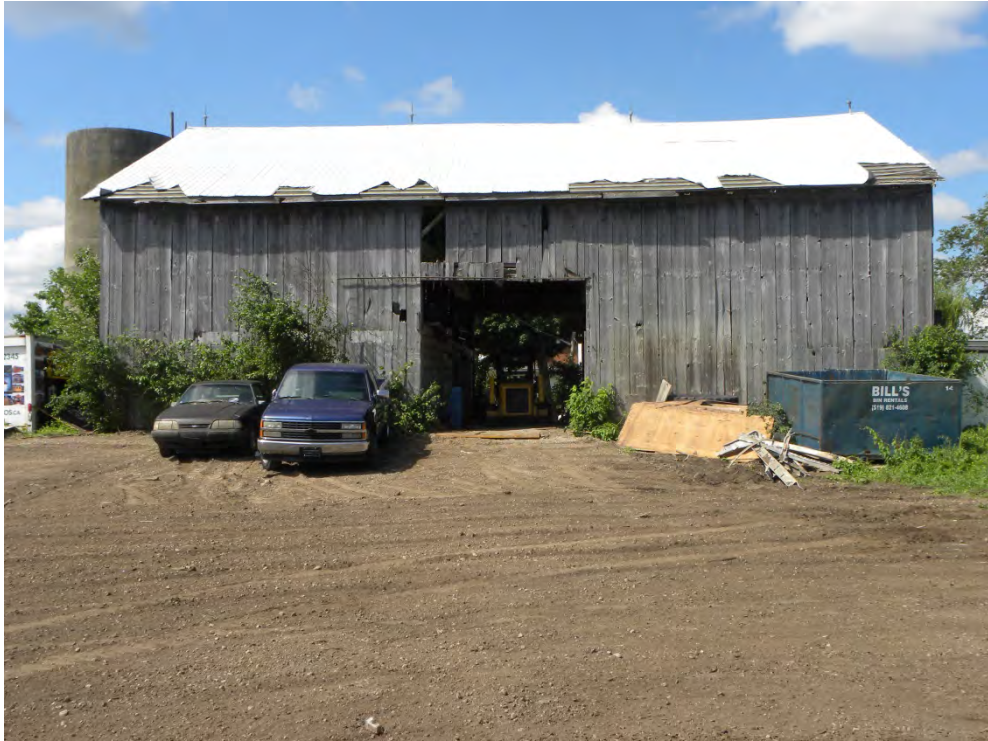
Plate 18: North façade of the barn showing three-bay arrangement of façade, with centered opening for wagon access
