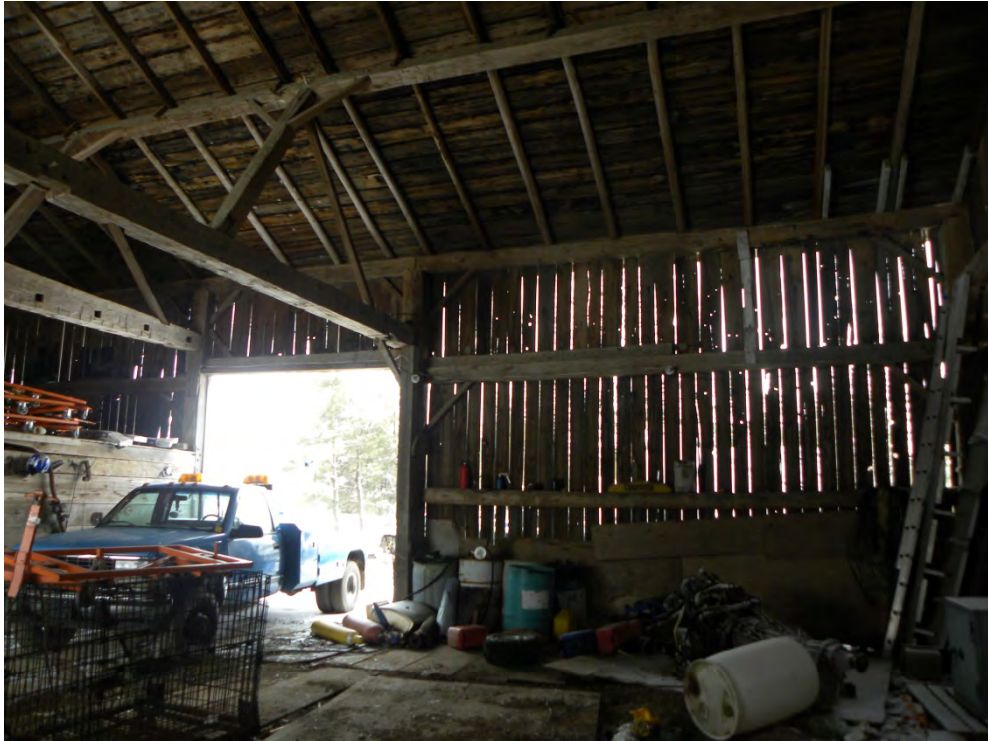
Plate 20: Interior south wall showing timber-frame construction of walls, posts and beams, and purlins supporting the roof
