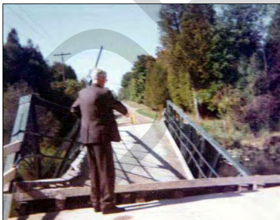
Figure 3. A view west depicts the collapsed Kortright Road Bridge, September 26, 1974 [City of Guelph].
