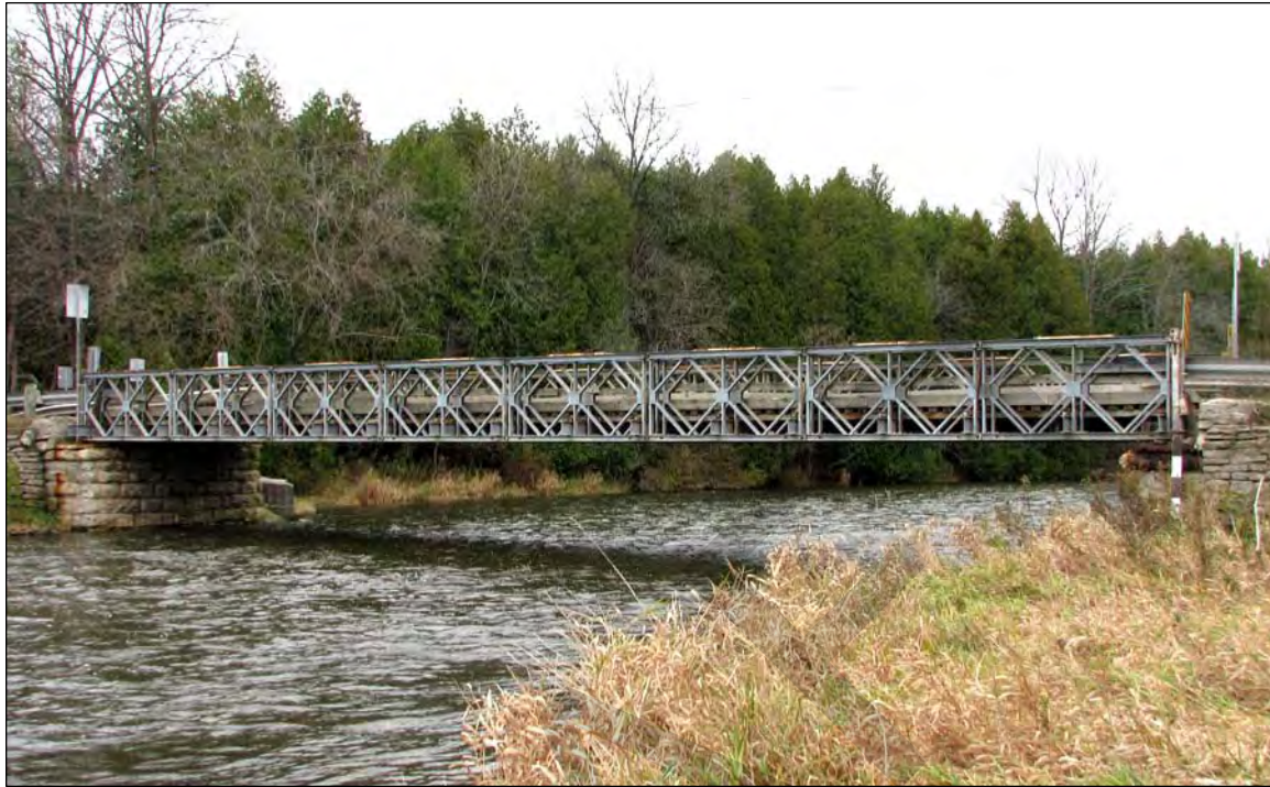
Figure 8. A view of the south elevation of the Niska Road Bridge depicts the Bailey bridge with stone abutments.
