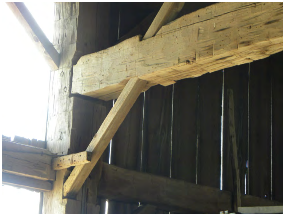
Plate 23: Tapered end of the swing beam that has been joined to the vertical posts using mortise and tenon joinery. The diagonal cross bracings have been replaced with modern dimensional lumber. Hewing marks are visible on the beam.
