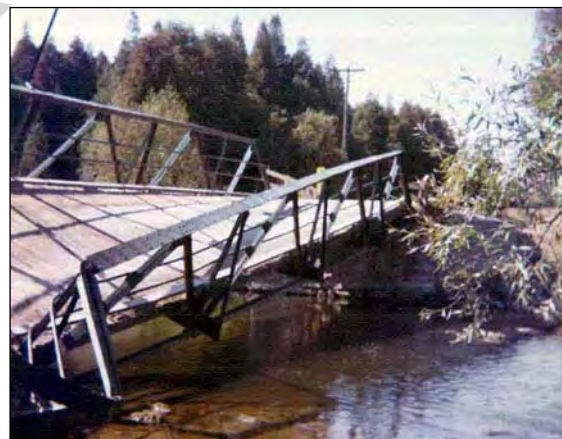
Figure 4. A view southwest shows the north side of the collapsed structure, September 26, 1974 [City of Guelph].
