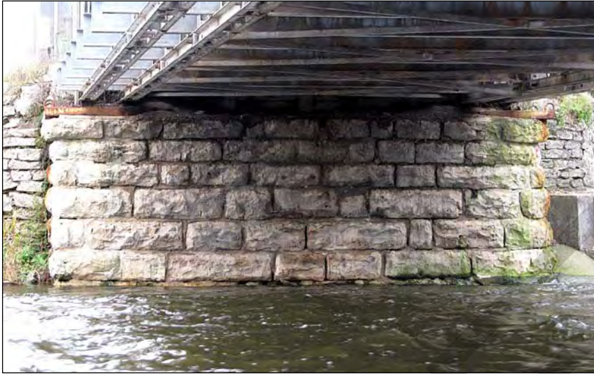
5. The abutments are faced in large dressed limestone blocks laid in six courses.
