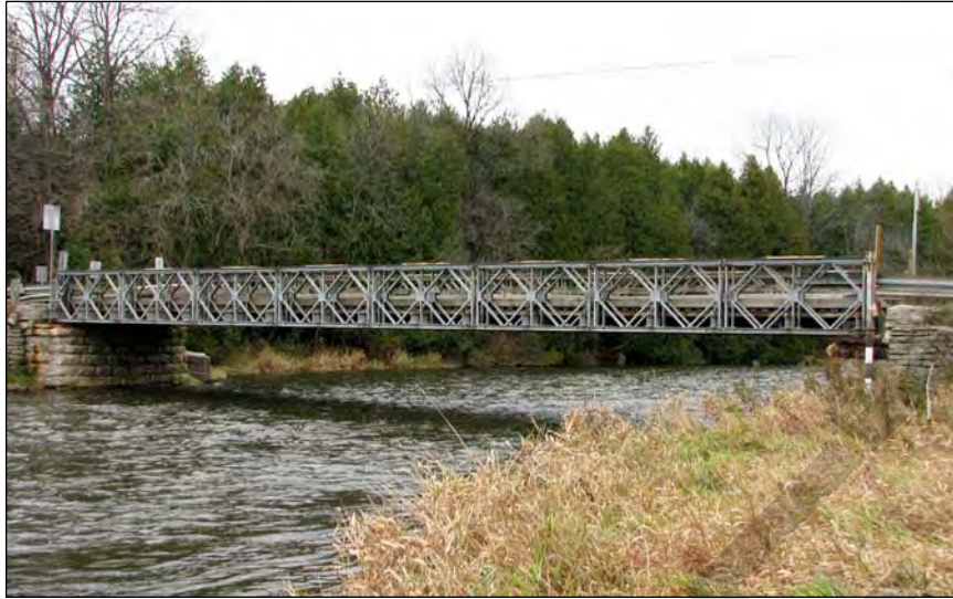
1. The Niska Road Bridge comprises a substructure of stone abutments and concrete rubble retaining walls and steel Bailey truss superstructure.
