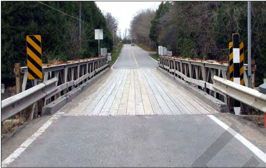
3. The Niska Road Bridge carries a single lane of traffic on a timber plank deck.
