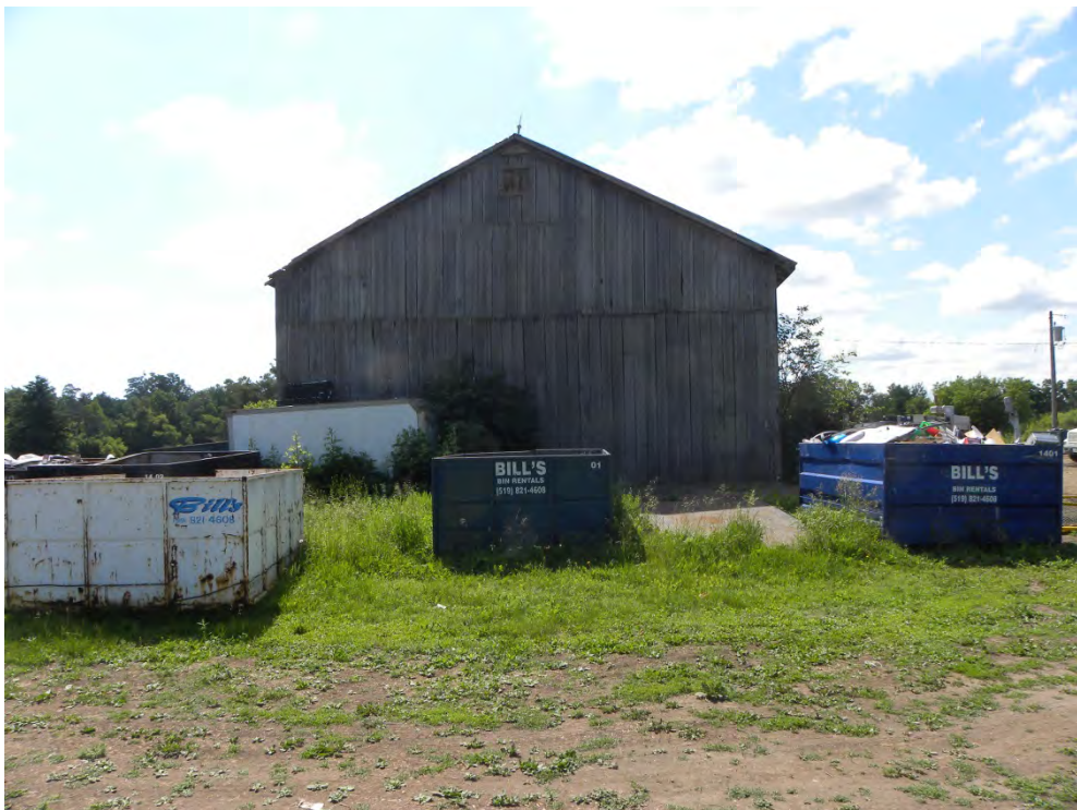
Plate 17: West façade of barn showing vertical pine plank siding, and low-pitched gable roof
