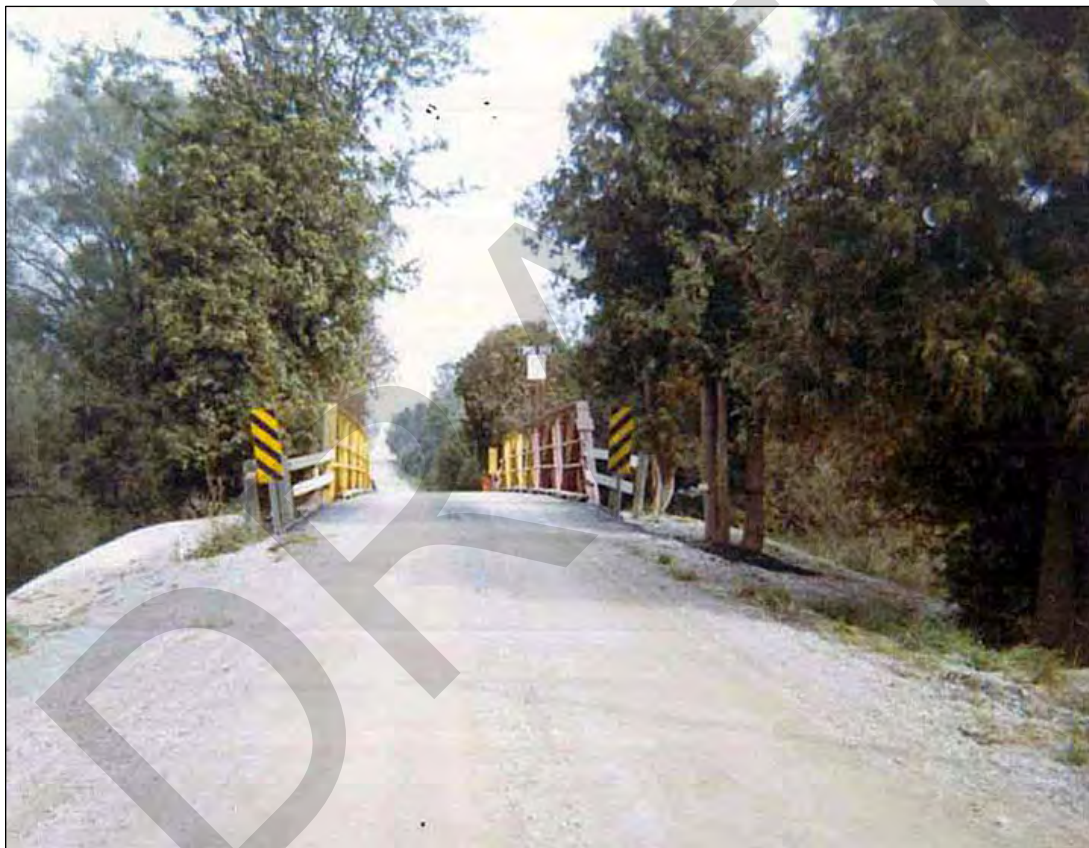
Figure 2. A view along the former Kortright Road shows the steel pony truss structure over the Speed River, September 20, 1971 [City of Guelph].
