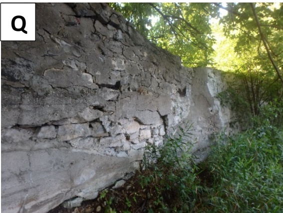
Condition of the existing east bank retaining wall upstream of Neeve Street
