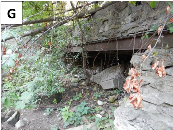
G Section of failed retaining wall and some potential retroactive structural stabilization (west bank)
