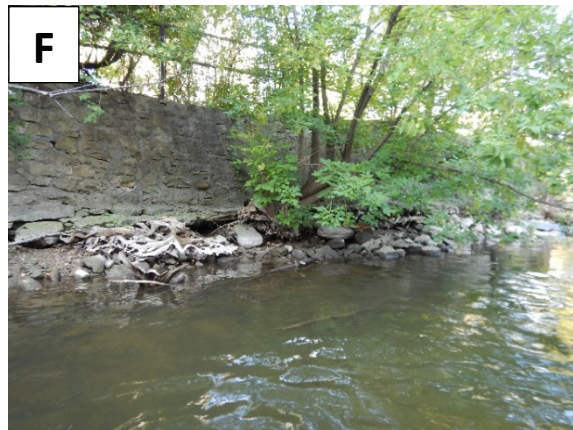
Looking at west bank where a tree was growing out of the retaining wall; this coincides with an approximately 2.4 m deep undercut.
