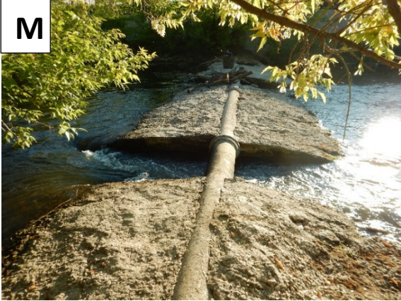
Looking east along sewer crossing; exposed pipe.
