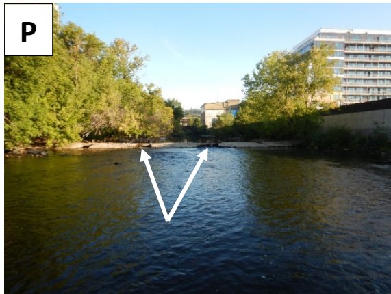
Looking upstream at the existing sewer crossing and pointing to the gaps between the concrete.
