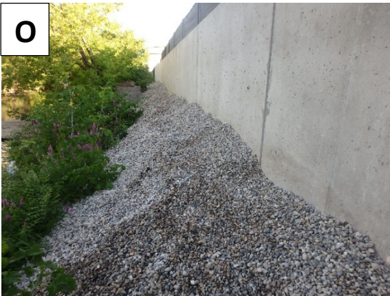
Section of east bank at sewer crossing. Gravel appears to have been placed at the toe of the recently constructed concrete wall.
