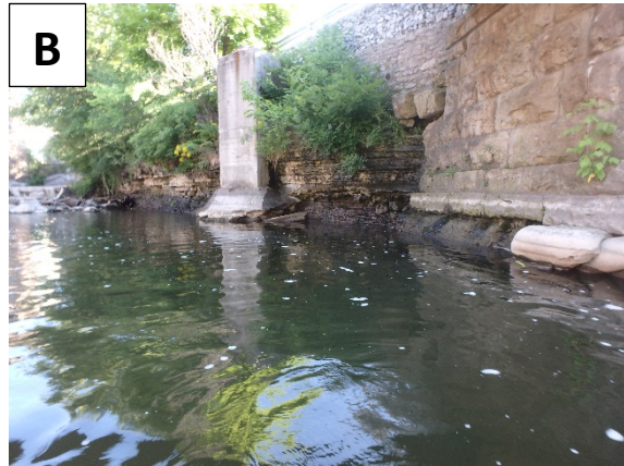
Sewer manhole structure situated along the east bank, between the CNR and GJR railway bridges; note the exposed bedrock surrounding the structure (interbedded shale and limestone/siltstone formations)
