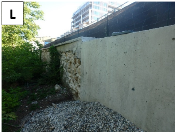
L Transition between old (repaired) and new (replaced) retaining wall on east bank upstream of sewer crossing.
