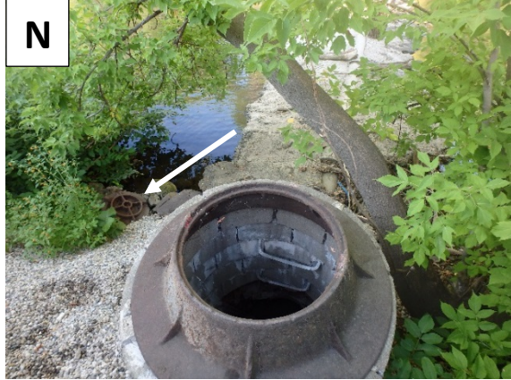
Sewer manhole at location of sewer crossing; note the manhole lid had been displaced. The lid was subsequently replaced by City staff.
