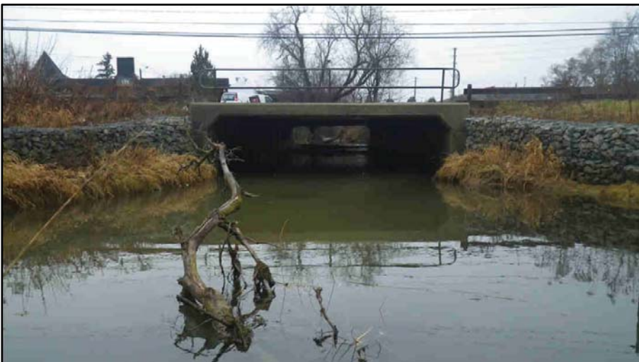
14. York Road crossing of Hadati Creek; structure is a concrete box culvert , gabion wing-walls protect the banks.
