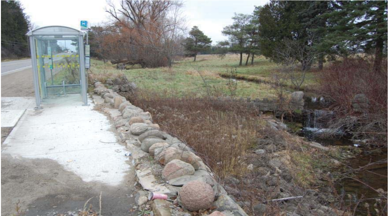
Photograph 1A: East side of entrance bridge. Only top of wall is visible.
