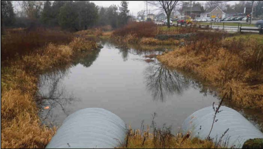
13. Two CSP culverts convey flows downstream from a parklands access road; channel immediately regains width downstream before Hadati Creek Confluence (background, right bank).
