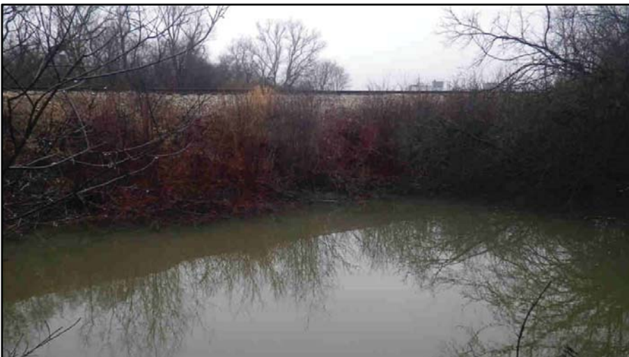
18. Clythe Creek flows immediately adjacent to railway embankment; embankment protection appears to be limited to vegetation. Water turbidity changes colour to appear more beige.
