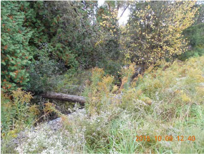
Gabion baskets next to roadway
