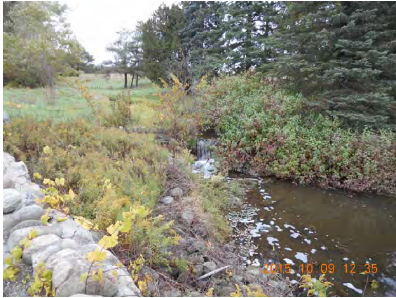
Cultural heritage wall and drop structure just west of former Reformatory driveway
