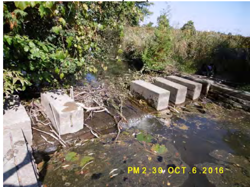
Damaged energy dissipation structure upstream of confluence with the Eramosa River
