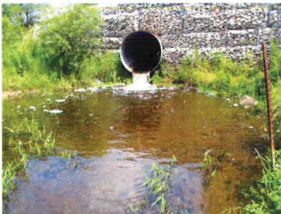
Photo 5: Perched culvert at Watson Road North (Site 4) presents a significant barrier to fish migration. Large schools of minnows (and minnow traps) can usually be observed in the pool below the culvert.
