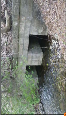
Feature 1: Alter to a concrete structure on the east side of the road. Feature 1 is located on the east side of the road.
