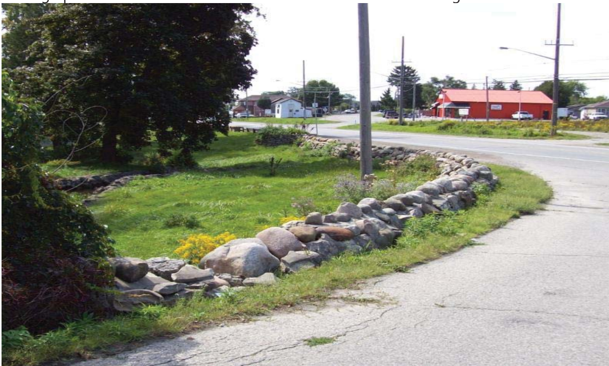
Photograph 4A: West of the entrance. Only the top of the wall is visible.
