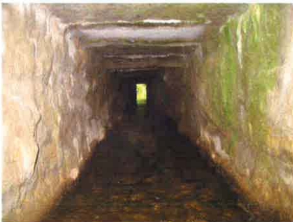
Photo 11: A long, dual-channelled, concrete culvert diverts the Creek from the north to the south side of the railway line.
