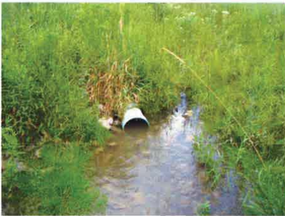
Photo 9: Discharge from the storm water pond was consistently turbid throughout the summer. Water quality in Clyde Creek was noticeably impacted and sedimentation of the Creek channel downstream of the pond outlet was observed.
