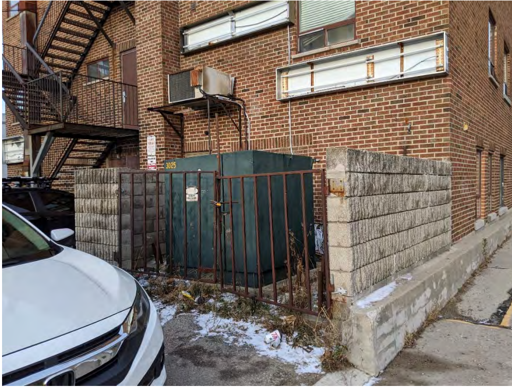
Photograph 9: Transformer located at 146 Wyndham (east of the Property)
