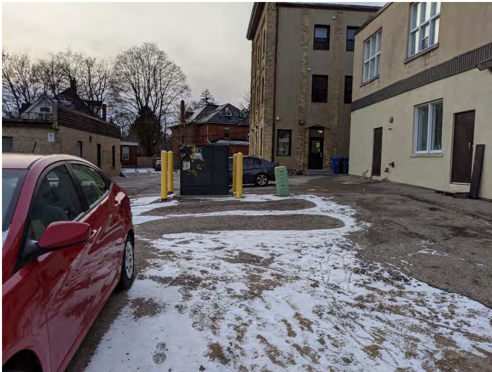
Photograph 10: Transformer located at 40 Baker Street (looking west of the Property)
