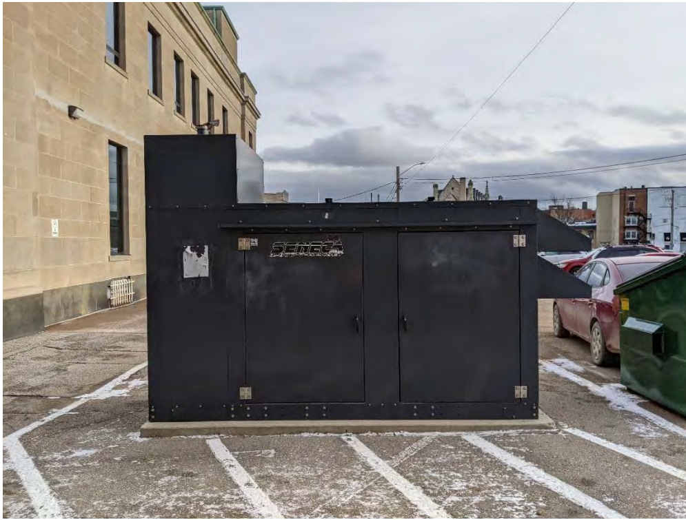
Photograph 1: Generator at 138 Wyndham, east of the Property
