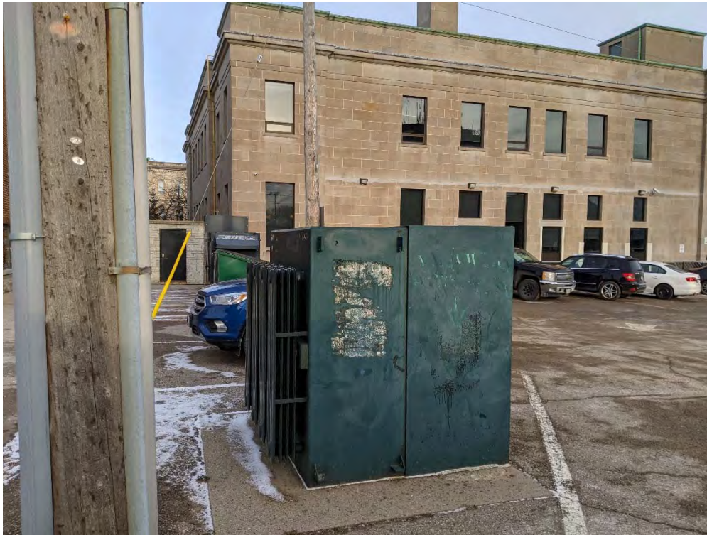
Photograph 11: Transformer behind 138 Wyndham Street (behind generator in Photo 1), east of the Property
