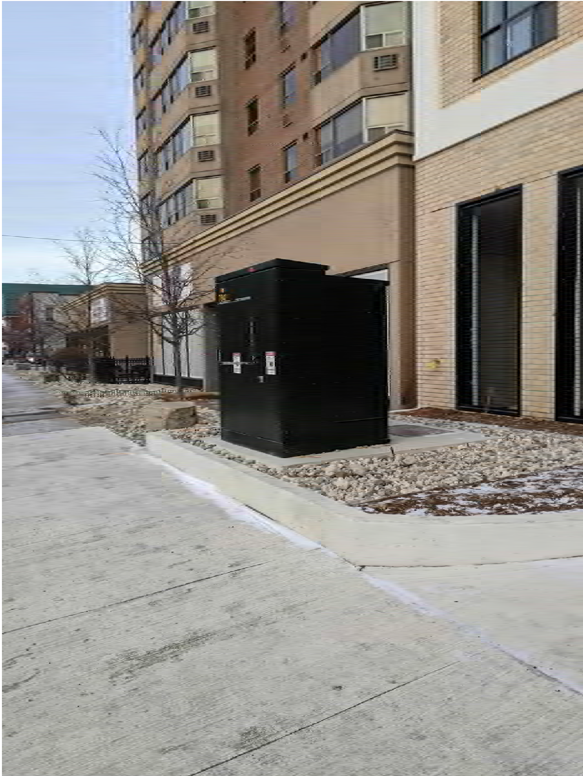
Photograph 8: New pad-mounted transformer located behind the building at 45 Yarmouth Street (west of the Property)
