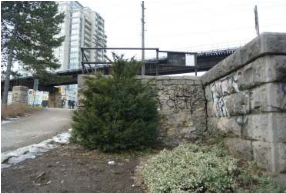
Plate 9: View toward the abutment of the former pedestrian bridge located to the south of the subject bridge.
