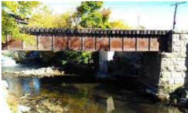
Plate 5: The Wellington Street Railway Bridge, looking north from the former Allan's Mills.
