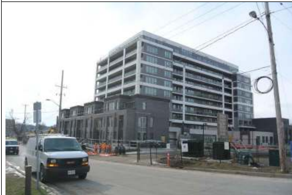
Plate 4: View southeast into the property from Arthur Street. Note the modern building in the process of construction.
