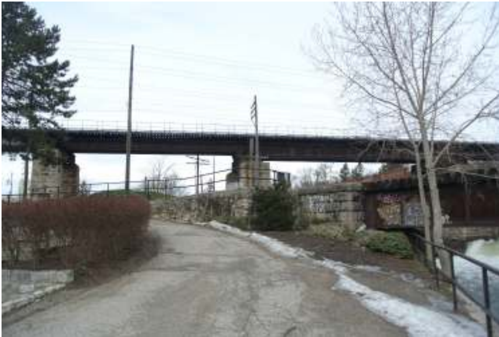
Plate 13: Detail of the stone retaining wall at the east abutment, looking north.
