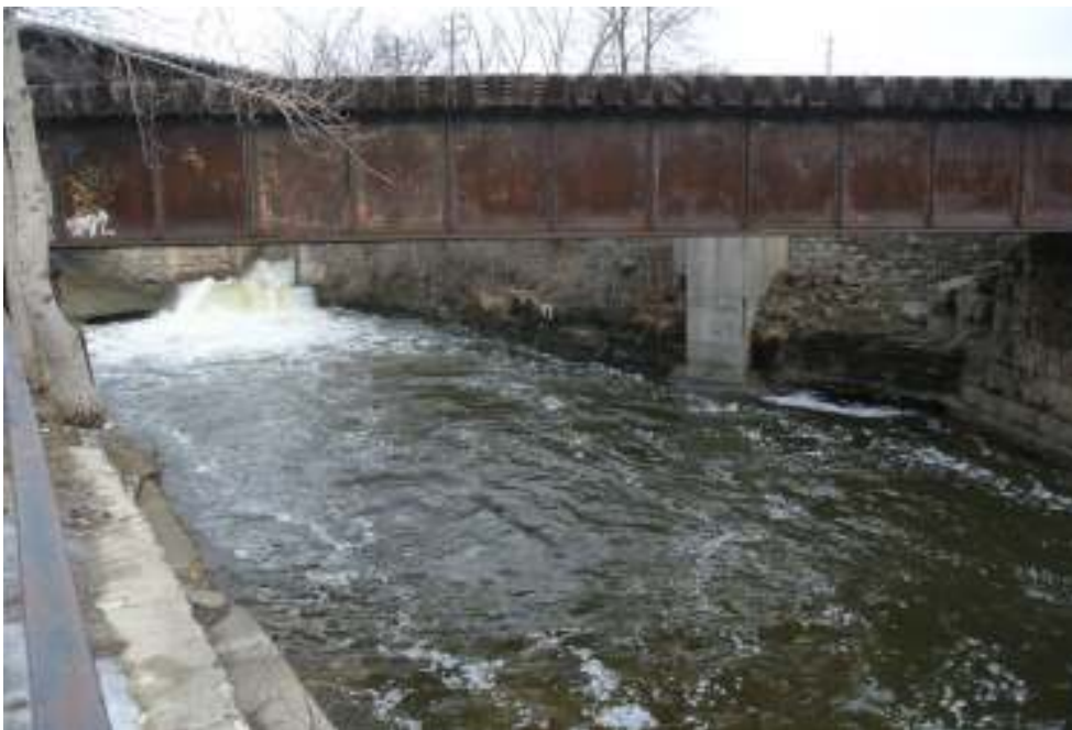
Plate 12: View toward the east abutment on the north side of the bridge. Note the stone retaining wall stretching north of the bridge.
