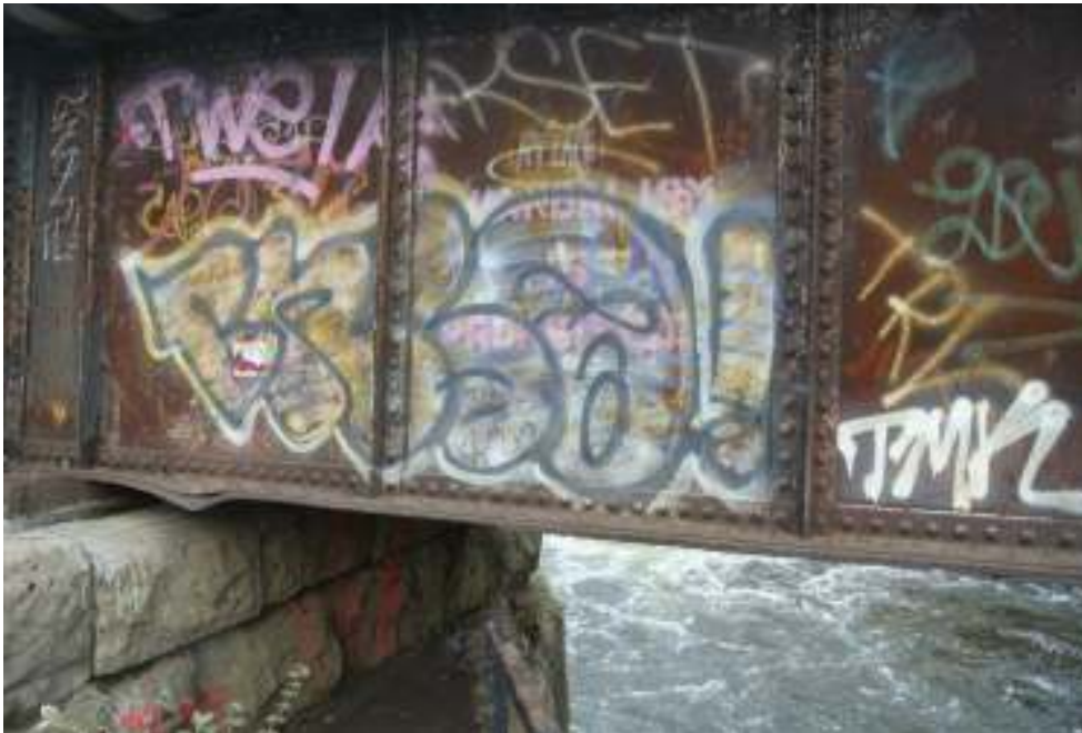
Plate 11: View toward the west abutment on the north side of the bridge, looking west.
