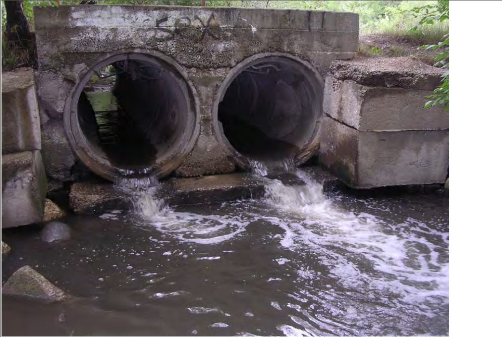
Photo 11: Perched twin culverts in Reach 4 inhibit fish passage. July 27, 2005.
