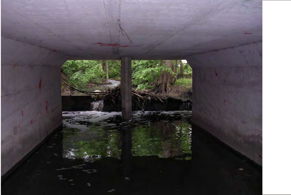
Photo 3: Barrier to upstream fish passage in Reach 1. July 27, 2005.
