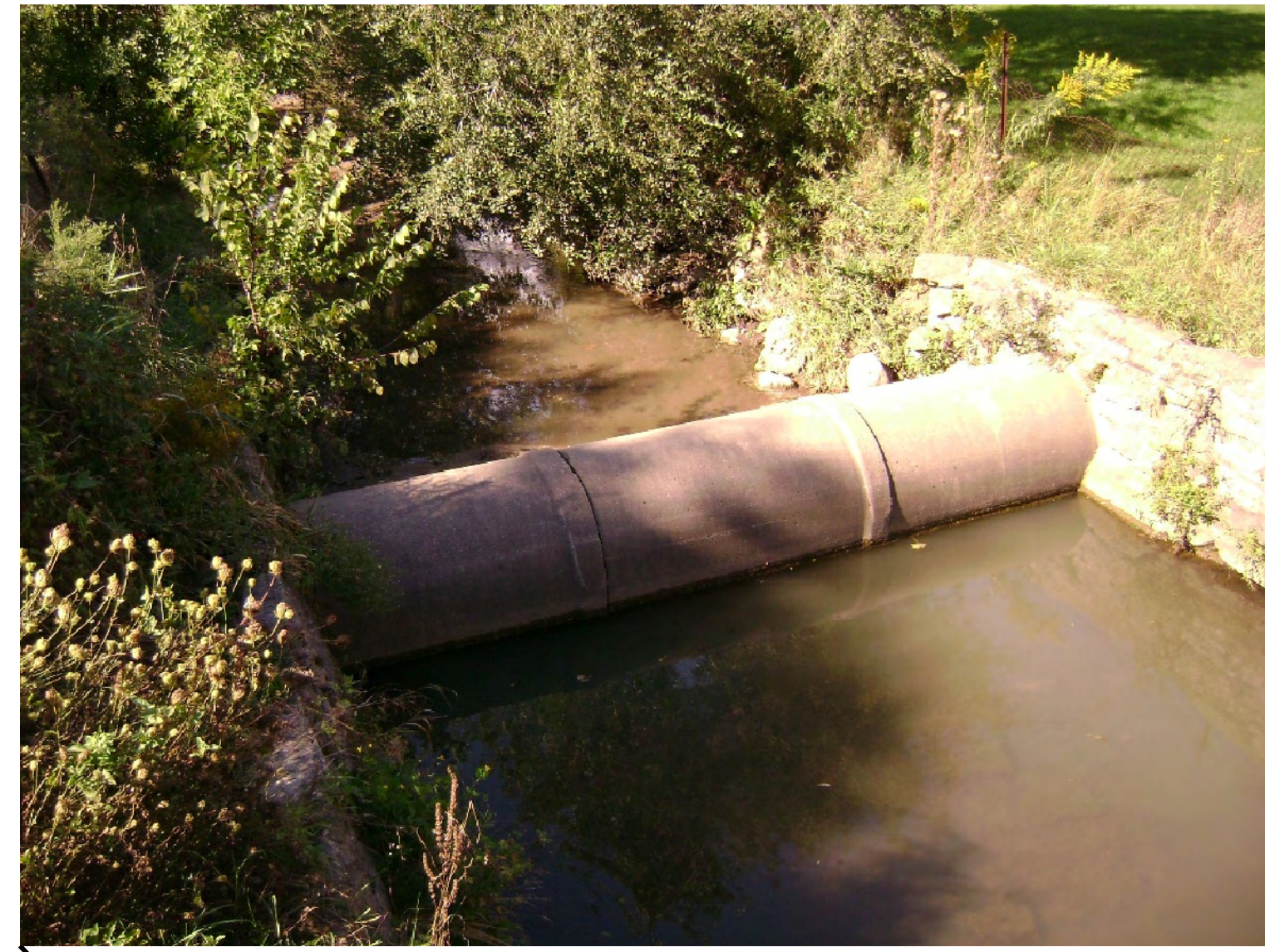
EXISTING YORK TRUNK SEWER CROSSING MUNICIPAL DRAIN IN SILVERCREEK PARK, BETWEEN EDINBURGH ROAD AND GORDON STREET
