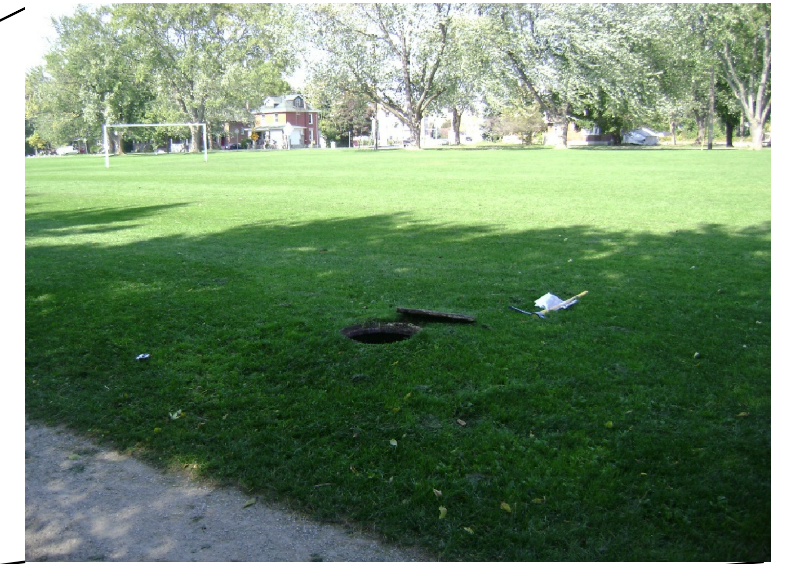
EXISTING YORK TRUNK SEWER ALIGNMENT ADJACENT TO SOCCER FIELD LOCATED IN YORK ROAD PARK
