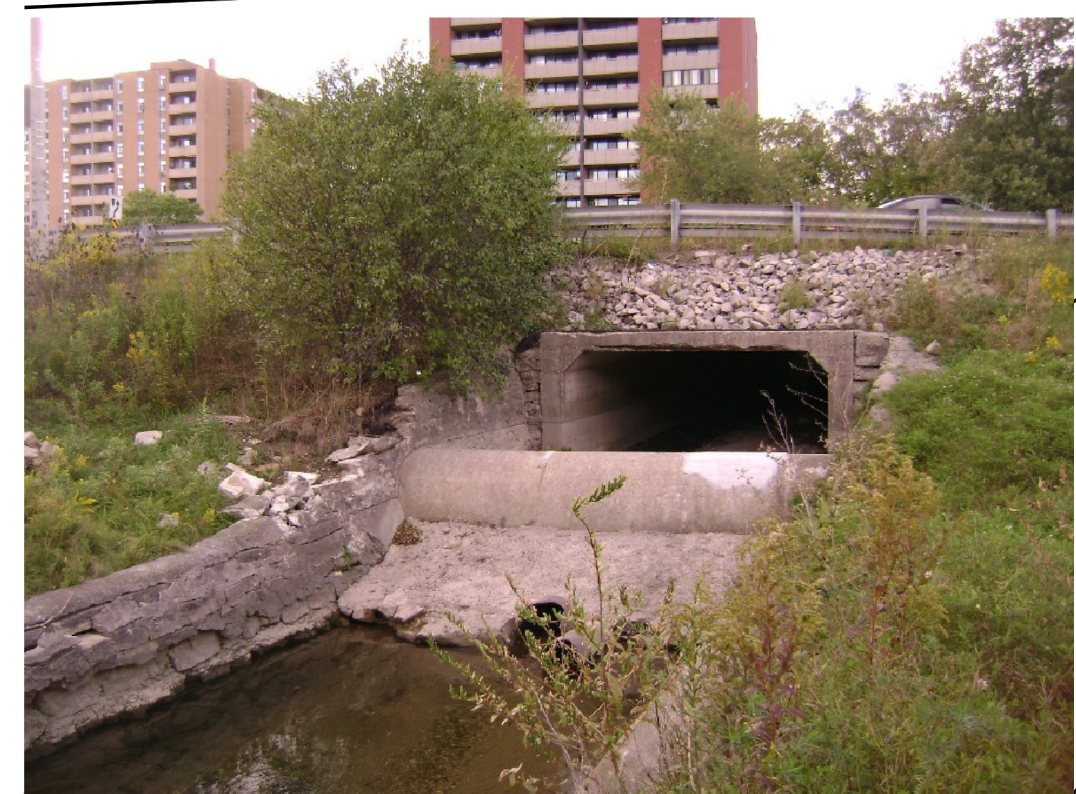
YORK TRUNK SEWER CROSSING MUNICIPAL DRAIN ON SOUTH SIDE OF WELLINGTON ROAD
